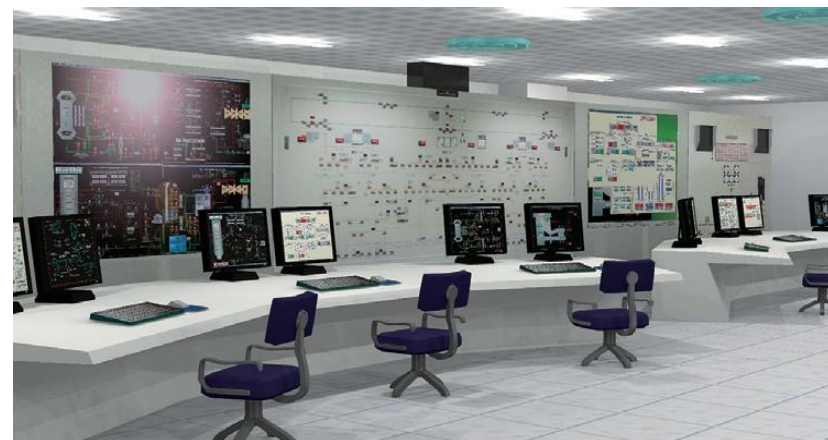
> CONTROL SYSTEMS & UPGRADES
