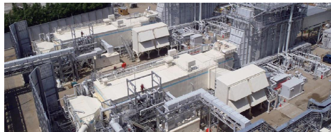
Client Tohoku Electric Power Co., Inc. Plant (country) Niigata Thermal Power Station Group 5 (Japan) Generating Power 109 MW Start Up 2011
