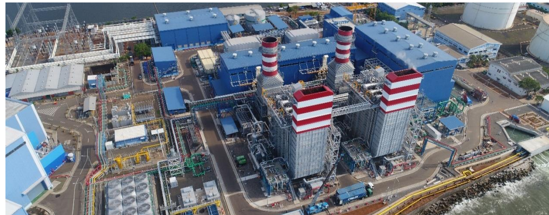
Client PT. PLN Plant (country) Tanjung Priok (Indonesia) Generating Power 880 MW Start Up 2019
