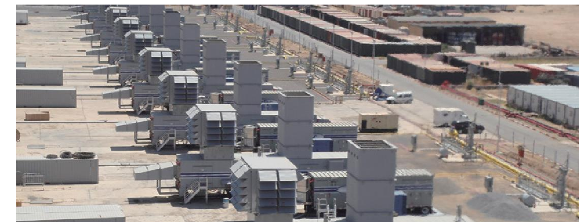
Client Sonelgaz Plant (country) Algeria Generating Power 1,350 MW (FT8MP x 54) Start Up 2011 / 2014 / 2015 / 2017
