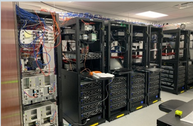
Netmation Protect Pack operational testing for multiple power blocks at Mitsubishi Power Cyberlab, Orlando,
